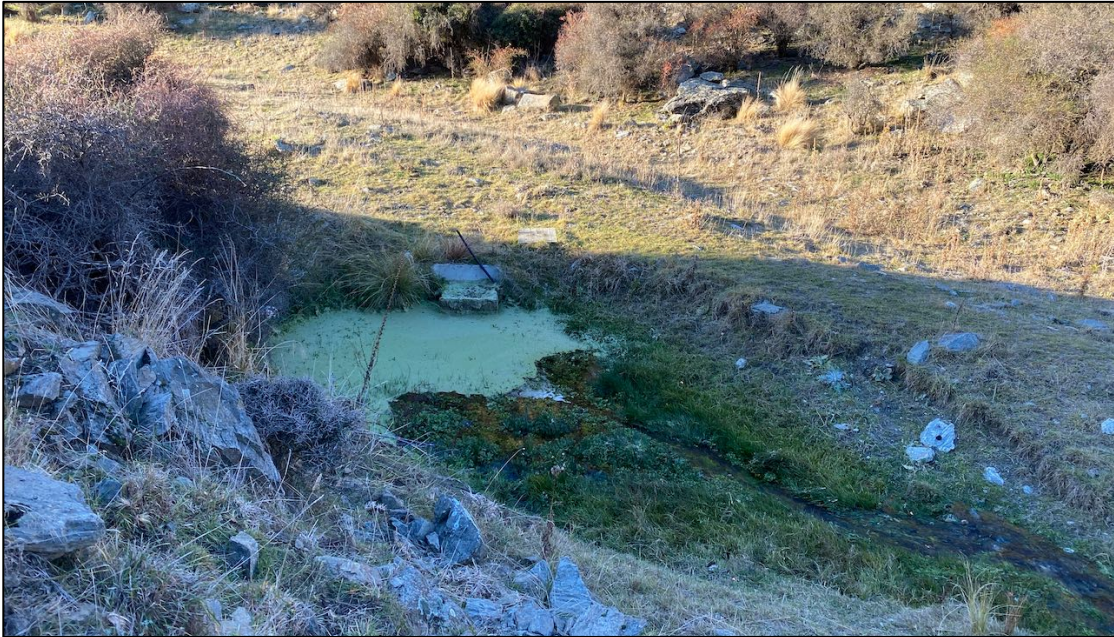
Figure 4: Lower Shepherds Creek irrigation weir at 100% capture.
