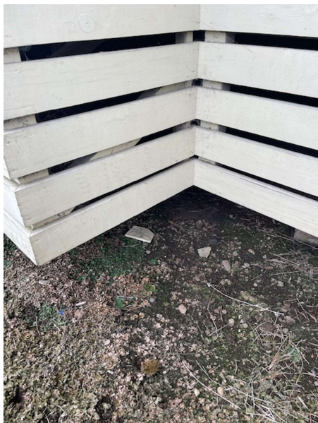
Photo 4: Suspected ACM debris
