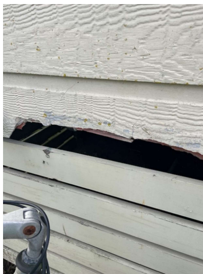
Photo 5: Suspected ACM cladding
