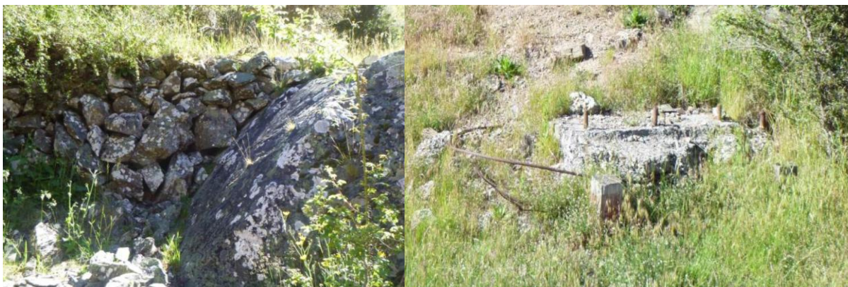
Figure 3: NZAA 2018 photos of revetted tramway (left image) and concrete machine foundations (right image)
