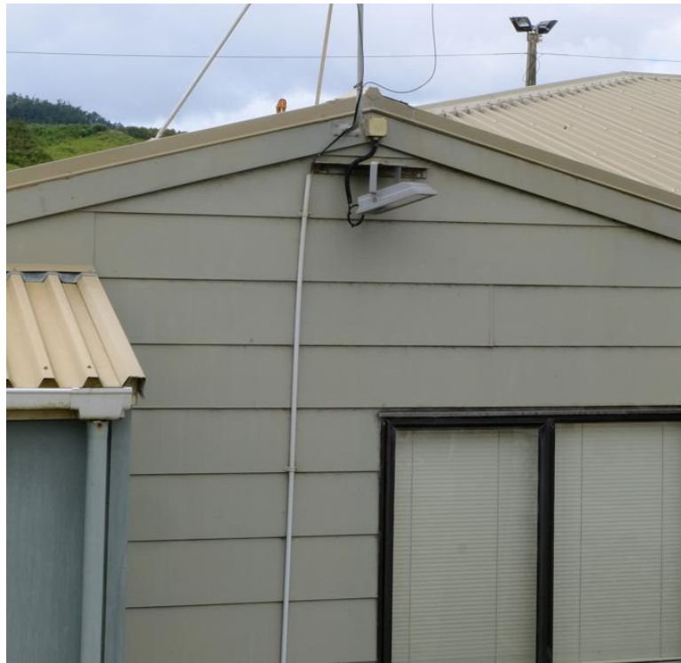
Figure 21: Typical Building Mounted Floodlight
