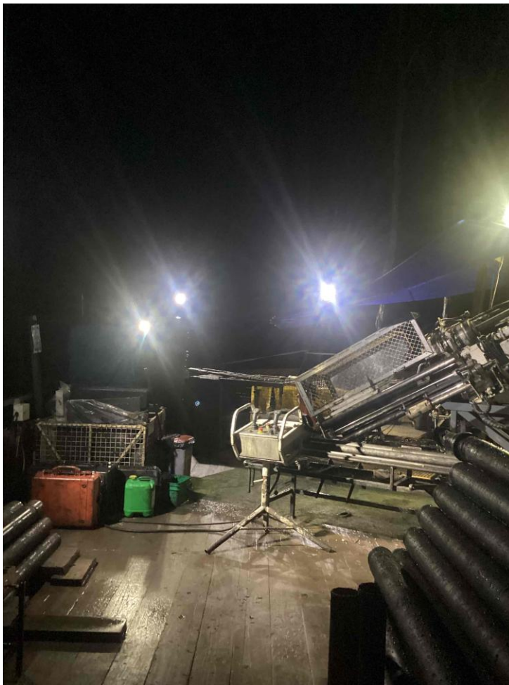
Figure 33: Drilling Site Lighting – Nighttime 1
