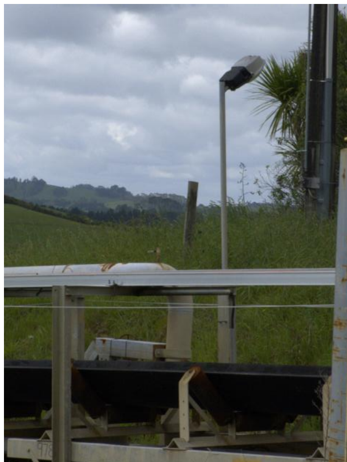
Figure 22: Conveyor Walkway Pole Mounted Bulkhead Luminaire
