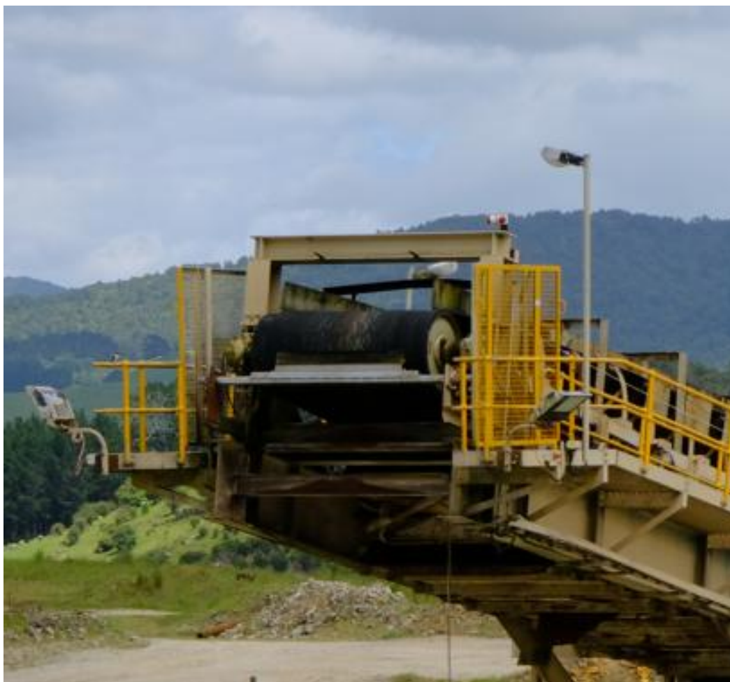
Figure 23: Conveyor Walkway Pole Mounted Bulkhead Luminaire 2
