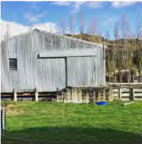
Sliding doors and external steps
