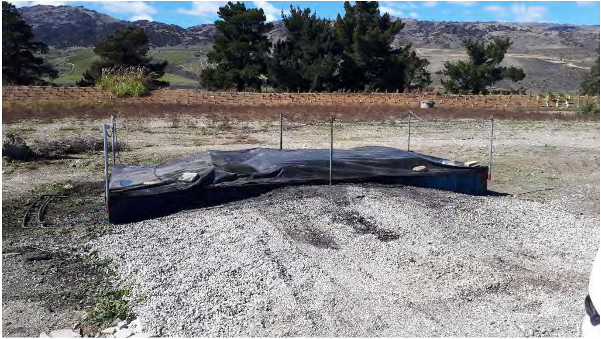
Figure 17: Road cutting waste storage.
