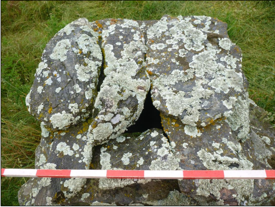
Figure 5 Photograph looking at top of chimney recorded as G41/678. Photograph taken by Phoebe Scrivener on 19/12/18.
