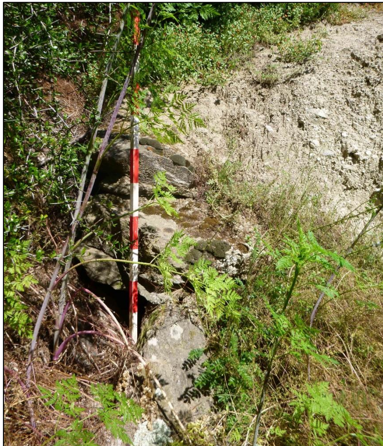
Figure 6. Photograph looking east at collapsed stacked schist culvert (POI 146).
