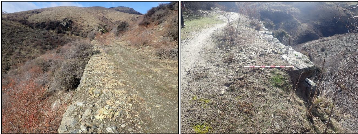
Figure 13. Photographs of stacked schist revetment (POI 810) southeast along the extent of the wall (left) and north (right) at the southeast end of the wall.
