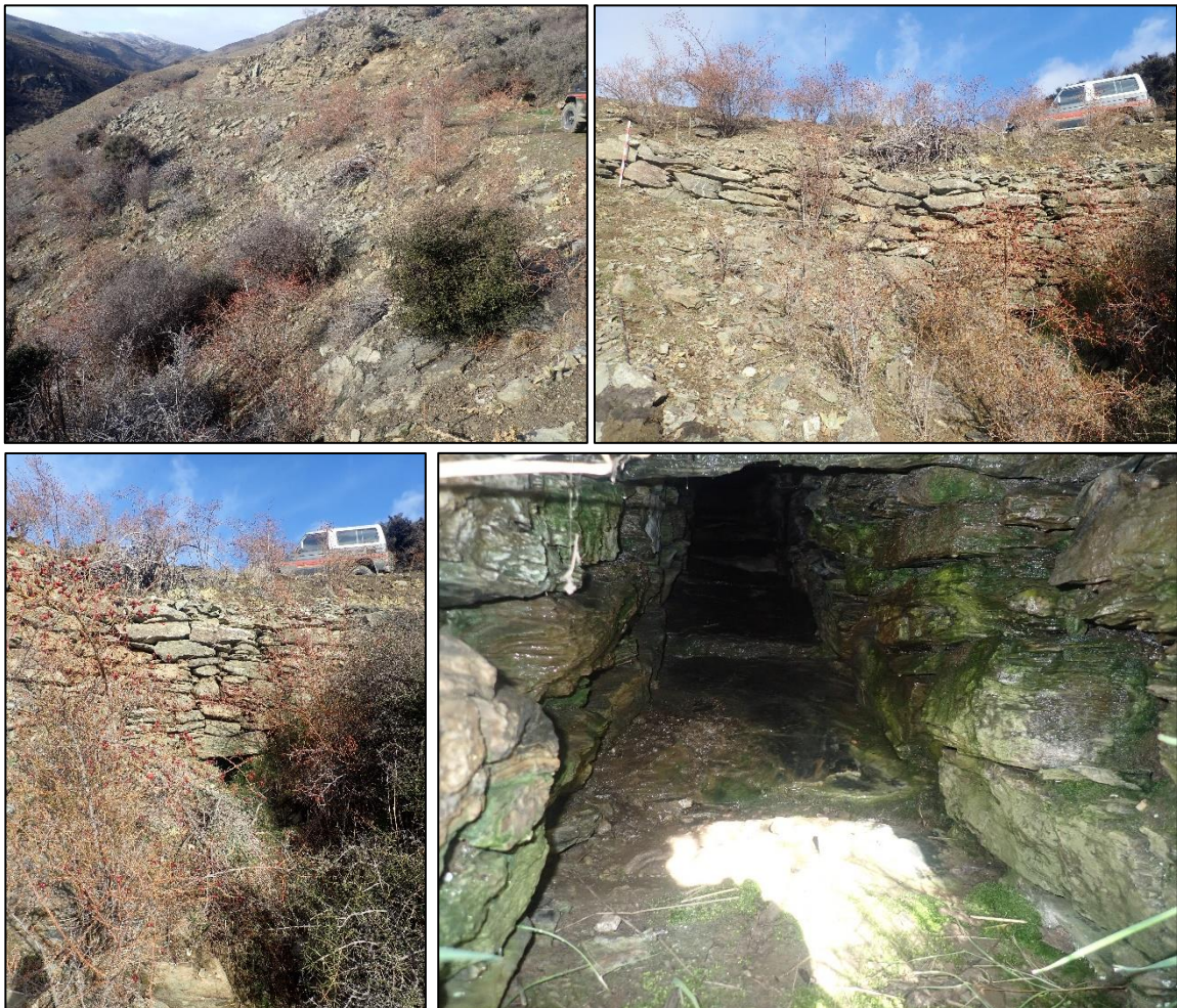
Figure 11. Photographs of culvert and revetment (POI 803) looking east (top left), north (top right), south at culvert (bottom left and right).
