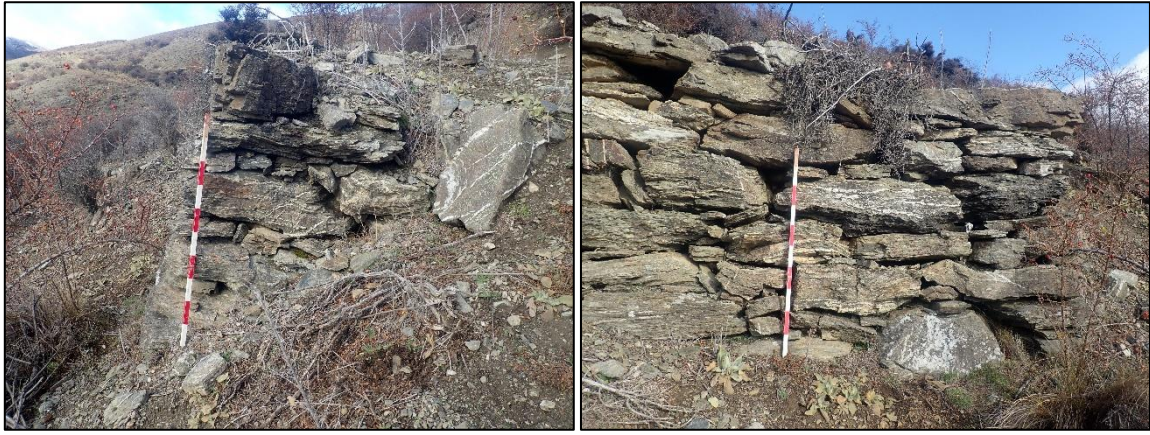
Figure 12. Photographs of stacked schist revetment (POI 810) looking southeast and southwest at the northwest end of the wall.
