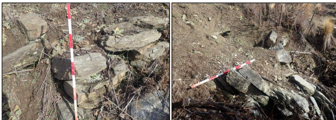
Figure 9. Photograph looking southwest at partial culvert (POI 798 – top left), collapsed culvert (POI 802 - top right)
