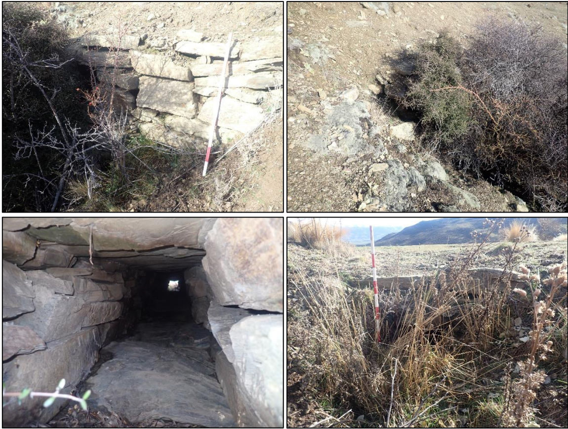
Figure 10. Photographs of culvert and revetment (POI 800) looking southeast at intact east end (top left), east at collapsed west end (top right), south at culvert (bottom left), and north at inlet (bottom right).
