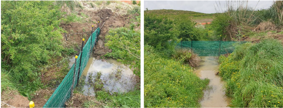
Photo 1 and 2. Photo examples of fish exclusion barriers
