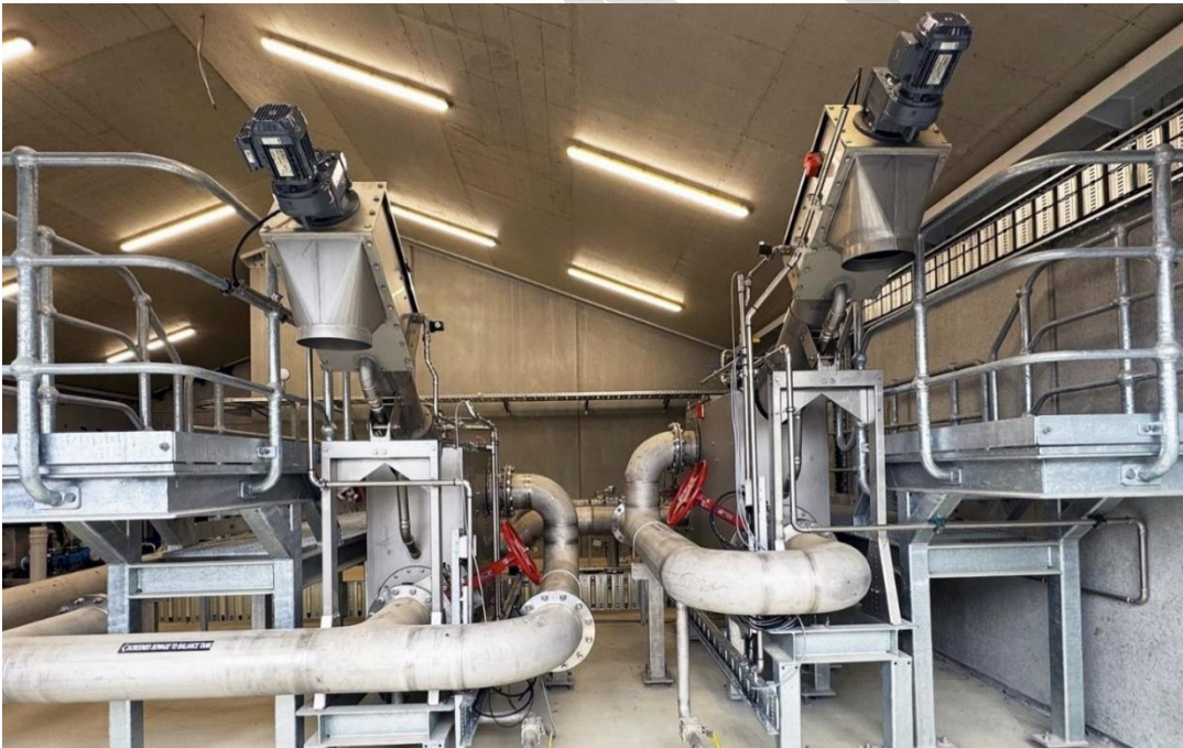
Figure 22: Inlet screening at Karaka North
