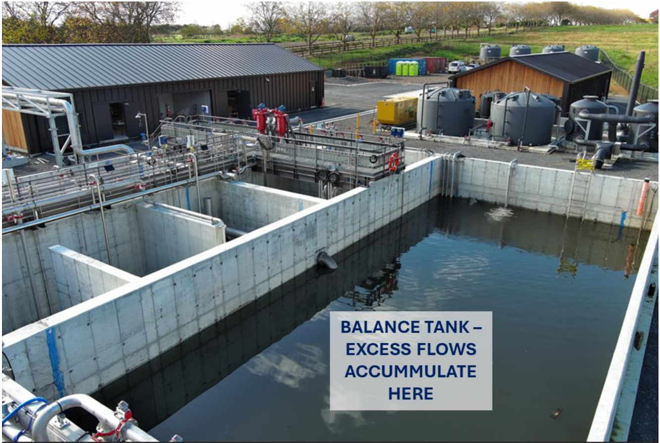
Figure 3: Karaka North WwTP flow balancing tank for MBR process
