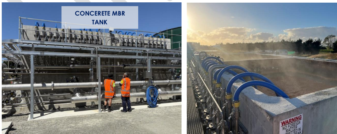
Figure 5: An Apex MBR membrane tank
