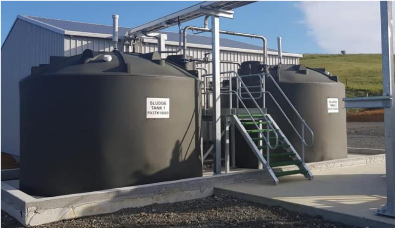
Figure 25: Example of sludge holding tanks at another WwTP
