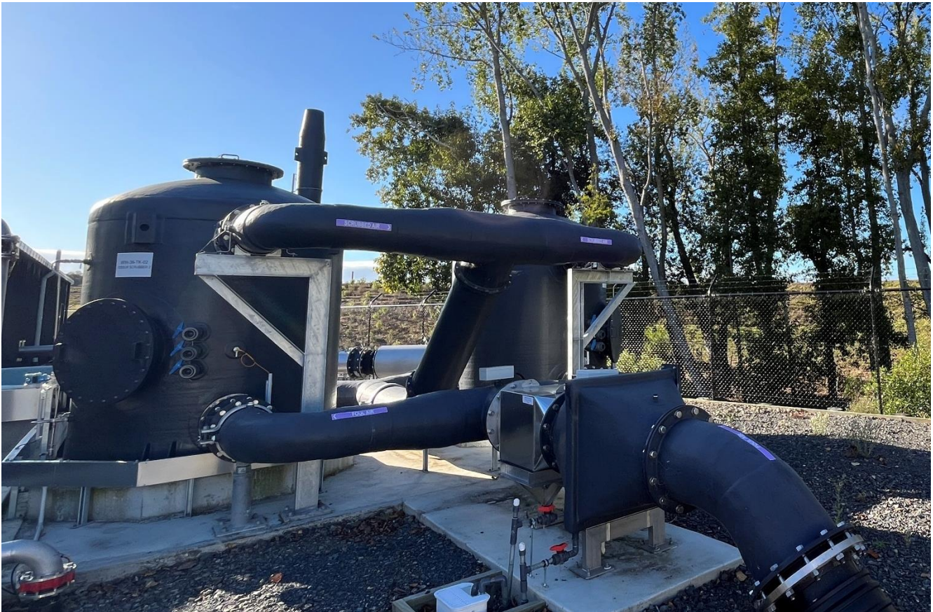
Figure 28: Activated Carbon odour control unit at Karaka North WwTP
