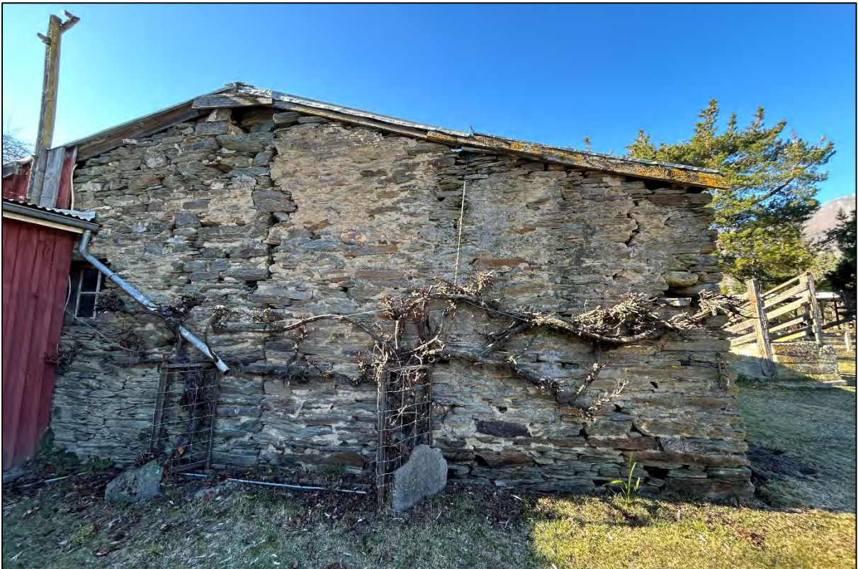
Figure 40. Western elevation of original stables, showing degradation and cracking.
