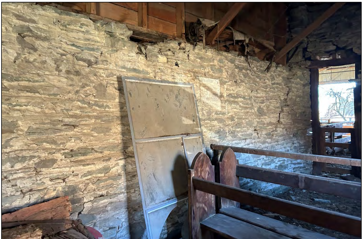
Figure 42. Internal woolshed wall showing degradation and lean.
