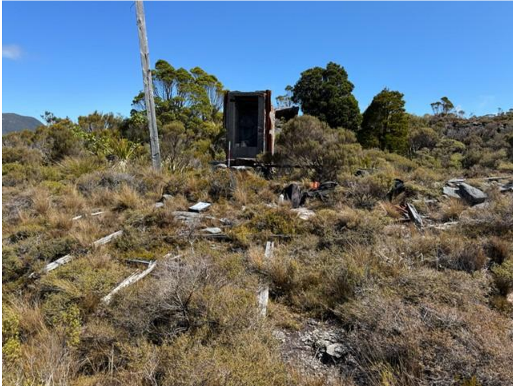
Figure 33. Collapsed remains of a building (corrugated iron and wooden beams) with a brick chimney on a stacked boulder foundation on Kiel's Flat. Standing power pole beside (Feature 119)
