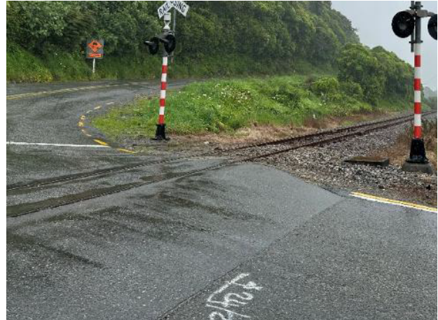
Figure 3-10: Small hump over crossing with gouge marks
