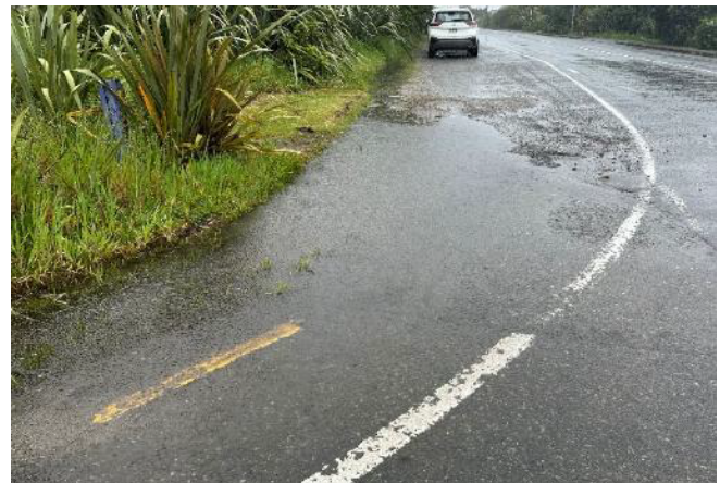
Figure 3-12: Water ponding on eastern side of road exiting into SH67
