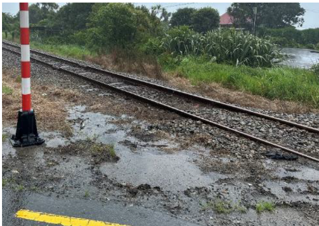
Figure 3-11: Water ponding on left side of road from eastern approach
