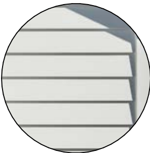
Bevel Back Weather Boards
