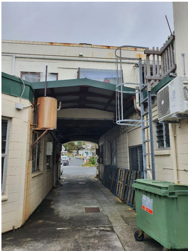
Photograph Appendix E.3: Above ground hot water cylinder was present at the rear of the drycleaners.
