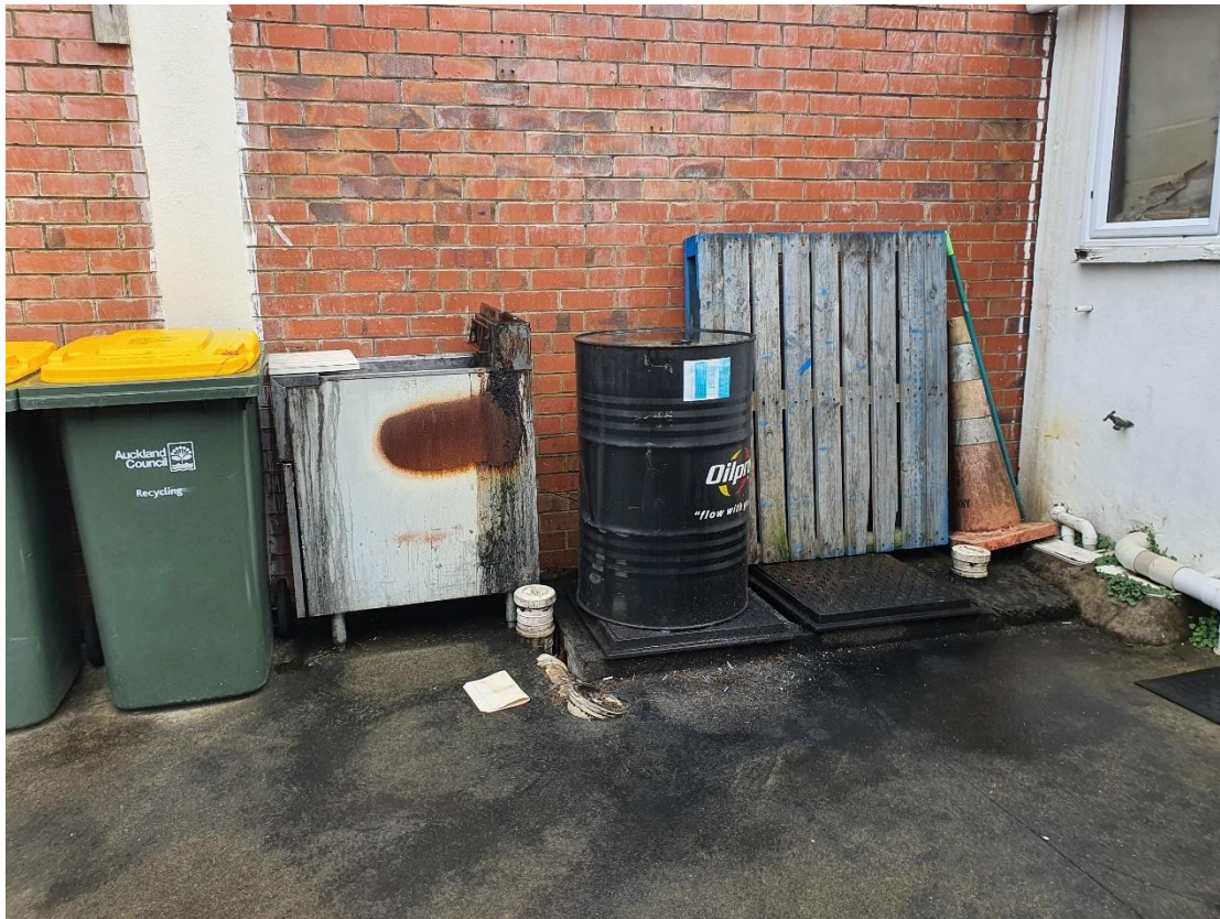
Photograph Appendix E.11: Grease trap interceptor and 200 L drum located at the rear of Victoria Road.
