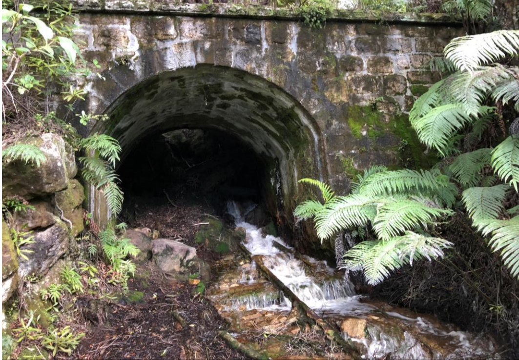
245 Figure 3-11: AMD-impacted groundwater discharging from an historic underground working into Miller Stream (source: BT Mining)
