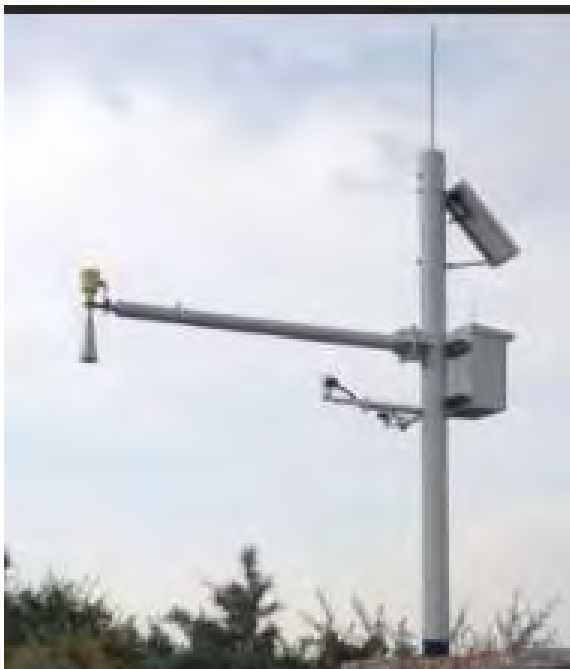
Figure 11: Example of rainfall and river level monitoring equipment
