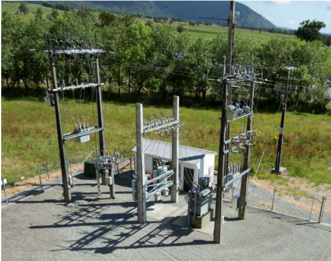
Figure 17: Example of Switching Station Equipment to be Included Within Westpower's Existing Waitaha Substation Site
