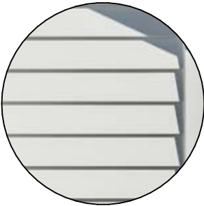
Bevel Back Weather Boards
