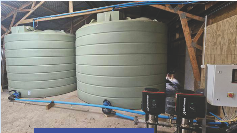
Figure 1 Installations at Waipapa
