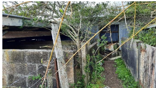
Photograph 8: Inside collapsed farm structure
