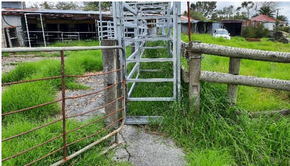
Photograph 5: Race and crush located on eastern side of the livestock farm structure
