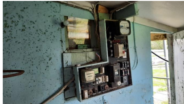
Photograph 6: Potential ACM, electrical backing board/panel
