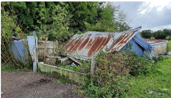
Photograph 7: Collapsed farm structure
