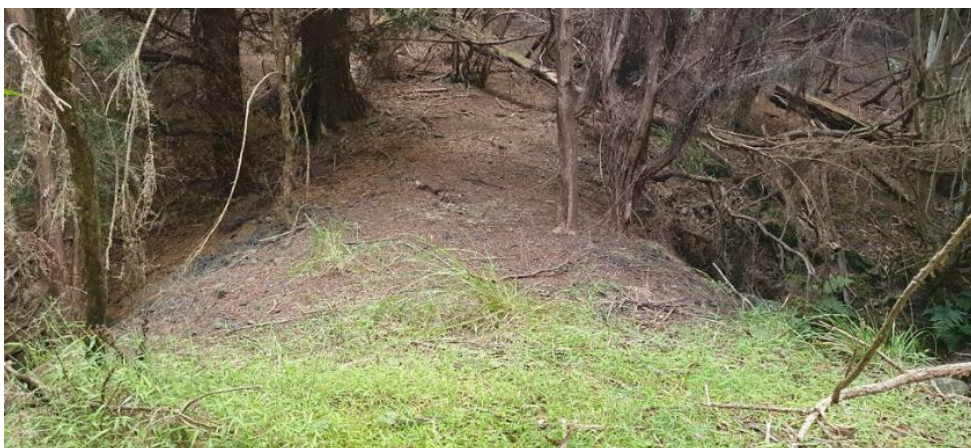
Figure 34. Photograph showing the land bridge over the top of a culvert in Area 2
