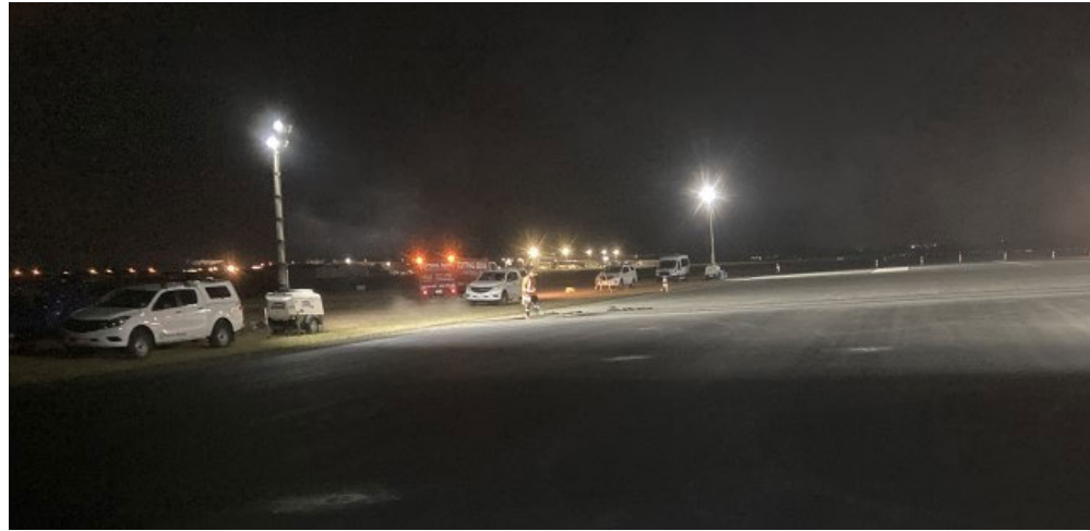
Figure 11: Typical Civil Works Mobile Lighting
