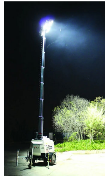
Figure 10: Typical Mobile Lighting Plant
