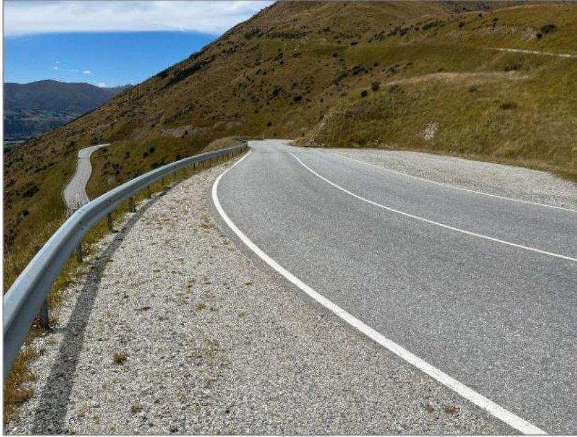
Figure 2-50: Typical view of Remarkables Ski Field sealed part of the access road.
