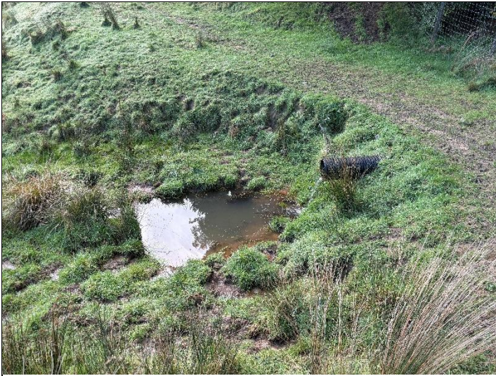
Upper end of main tributary with perched track culvert.
