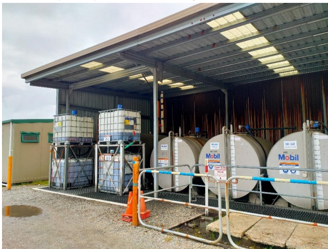
Figure 6.2: Bulk oil tanks and packages of oils at the workshop, undercover and within a bund.
