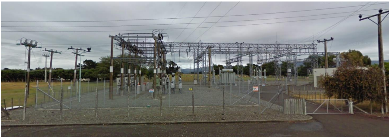
Figure 4: Existing Greytown Substation on Bidwills Cutting Road (Google Streetview)
