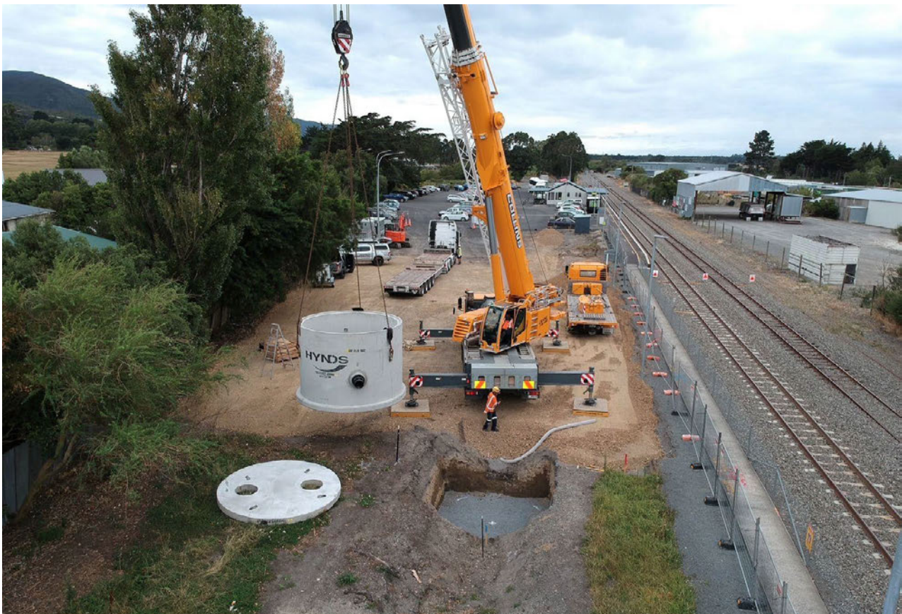
Fig. 5 18 module Up-Flo inside a 3.0m dia manhole treating a 6,500m2 carpark at Featherston Railway station. Credit SDCI for image.
