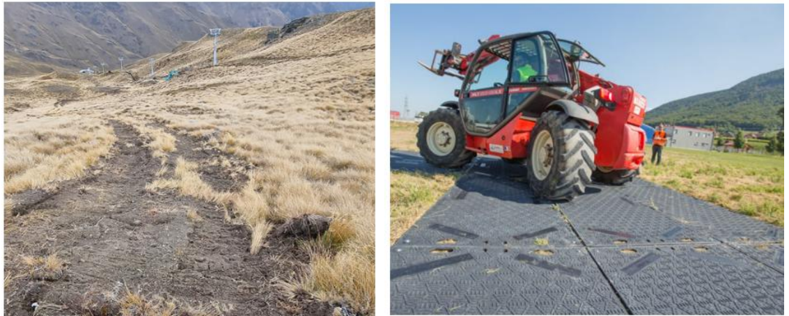
Figure 3-27: Example of temporary access track (left), rubber matting for use near critical source areas (right).
