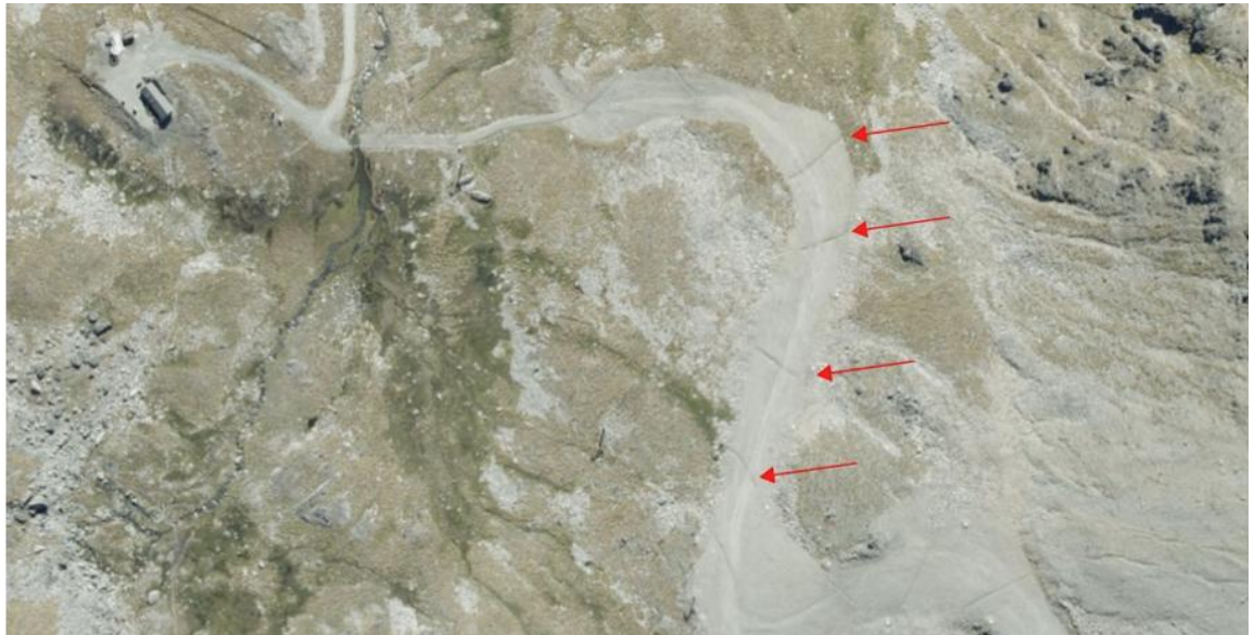
Figure 3-23: Stormwater channels to maintain surface sheet flow as much as possible, as used in the Rastus Burn catchment (Stantec, 2026d).
