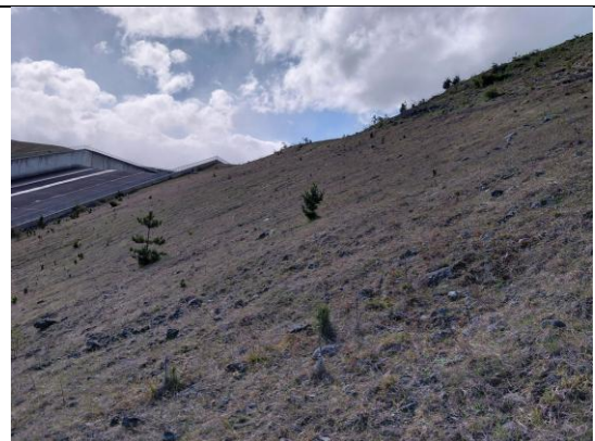
Photograph Appendix D.8: Mackenzie skink habitat on the batter to the Lake Pūkaki dam spillway. Habitat comprised short grasses, boulders and cobble piles to ~0.75-1 m depth.
