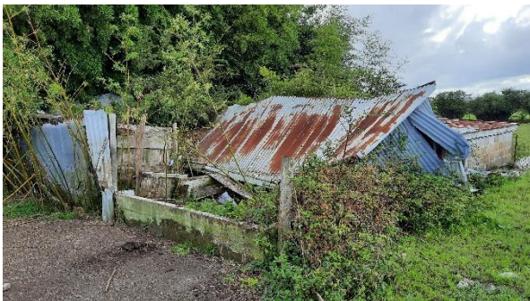
Photograph 7: Collapsed farm structure
