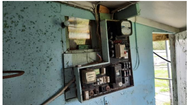
Photograph 6: Potential ACM, electrical backing board/panel
