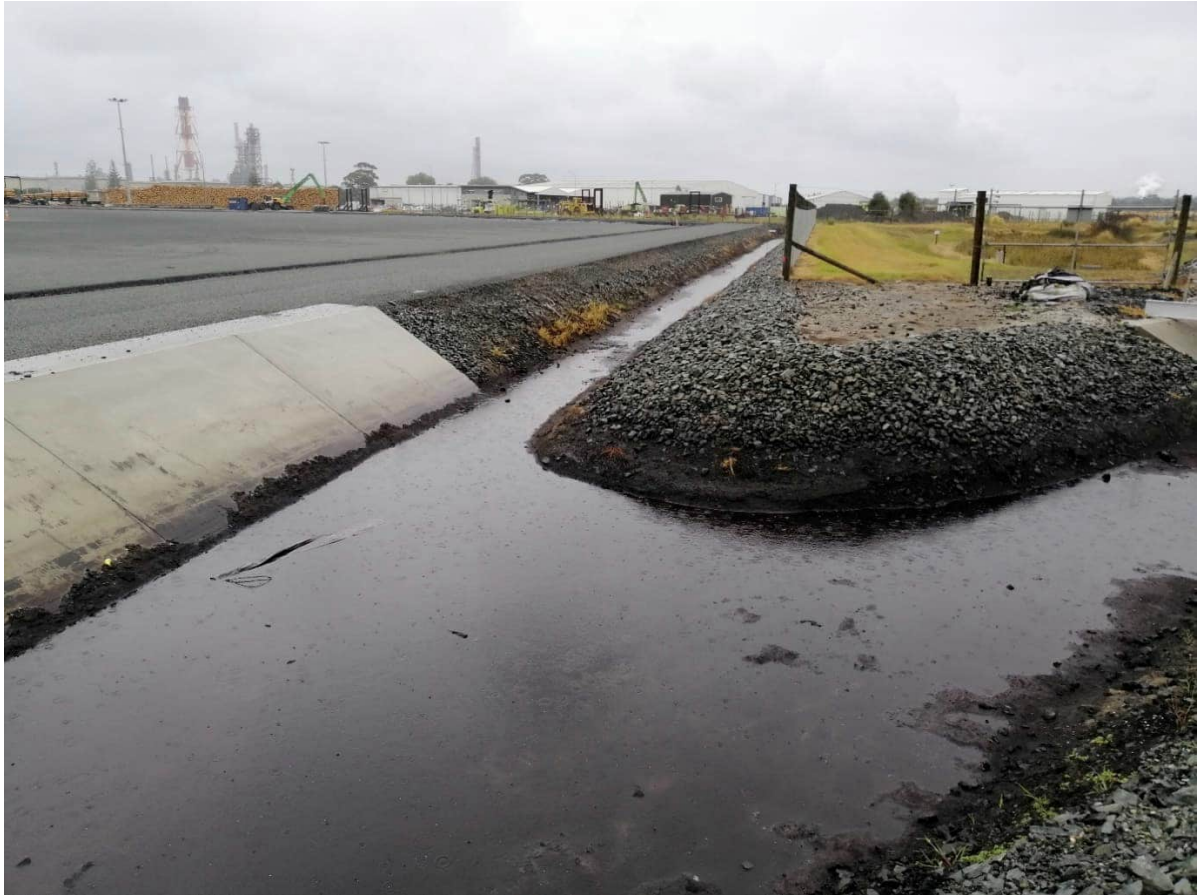
Figure C: Typical Northport collection and conveyance canal. Note runoff from the port apron is for the most part direct discharge as lateral sheet flow.
