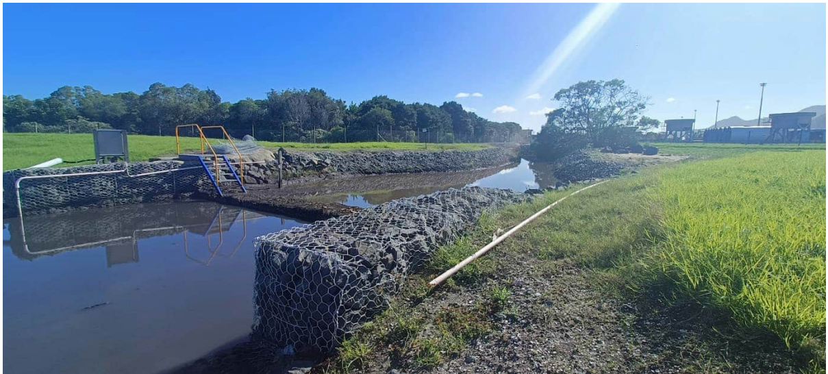
Figure E: Northport treatment pond inlet weir from the canal system elevated water level condition – view N approx.
