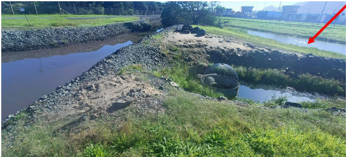
Figure H: MMH Industrial treatment pond overflow and reach to pond outlet (arrowed) with Northport pond inlet canal on LHS
