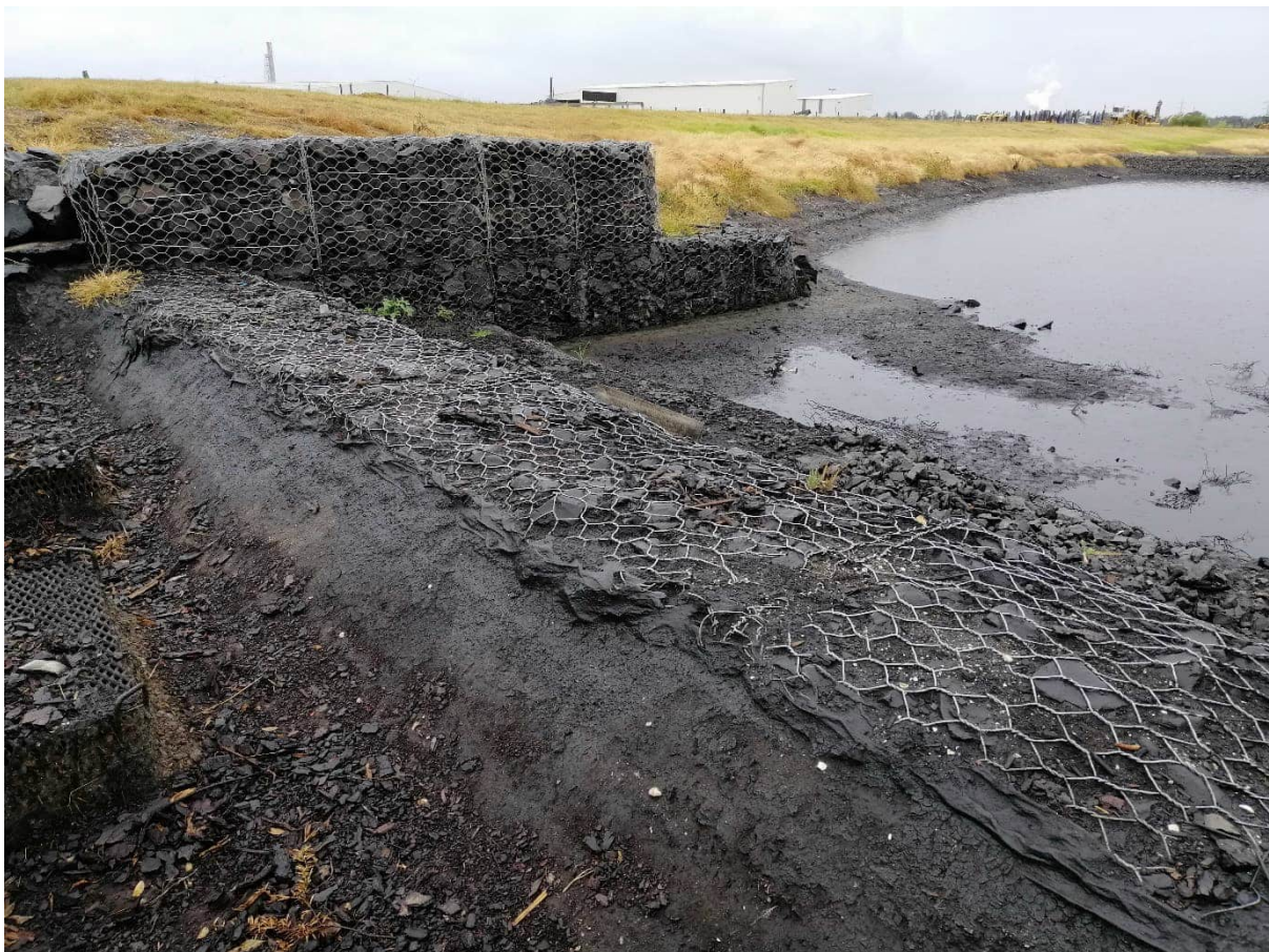
Figure G: Northport treatment pond inlet weir at low water level – view SSE approx.
