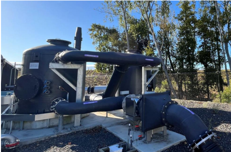
Figure 17: Activated Carbon odour control unit at Karaka North WWTP
