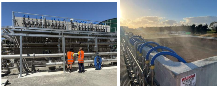
Figure 9: Apex MBR membrane tank
