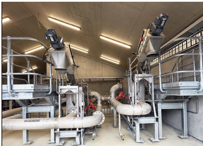
Figure 14: Fine and Coarse Inlet Screens at a treatment plant designed and built by Apex Water
