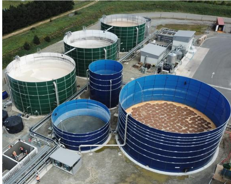
Figure 15: Operating aeration tank (Large Blue Tank)
