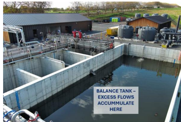
Figure 7: Karaka North WWTP flow balancing tank for MBR process
