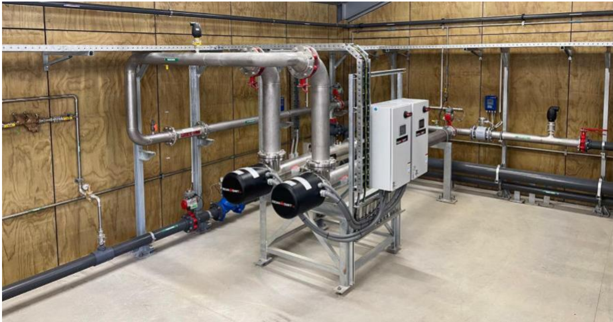
Figure 4: Duty / standby UV disinfection units (Karaka Village North WTP)
