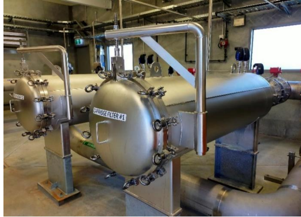
Figure 2: Duty / standby cartridge filter units (Motueka WTP)
