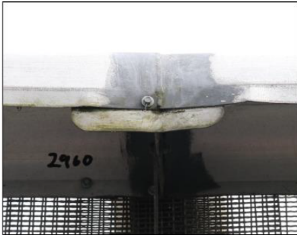
Image 1: Zinc blasted welded joint on the fence hood.
