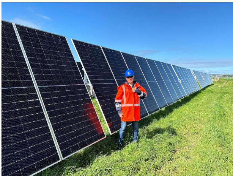
Plate 1. Single axis tracker photovoltaic panel design.
