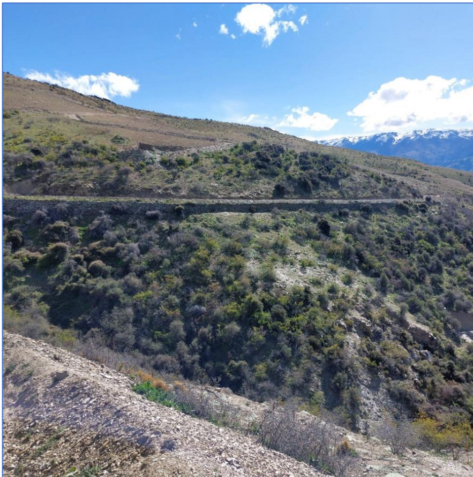
Figure 10: View into a section G41/782 historic carriageway - damaged by conversion to mine access.
