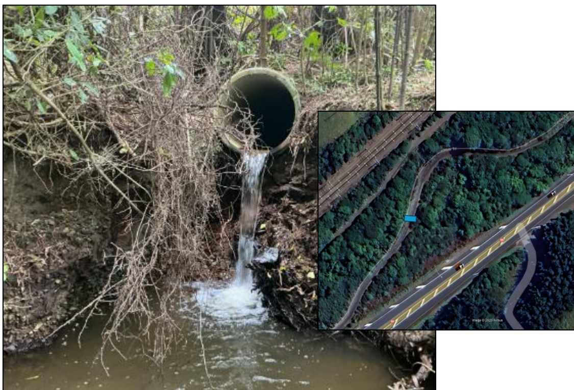
Figure 14. Lower walking track culvert entrance - a fish barrier (inset shows approximate location).
