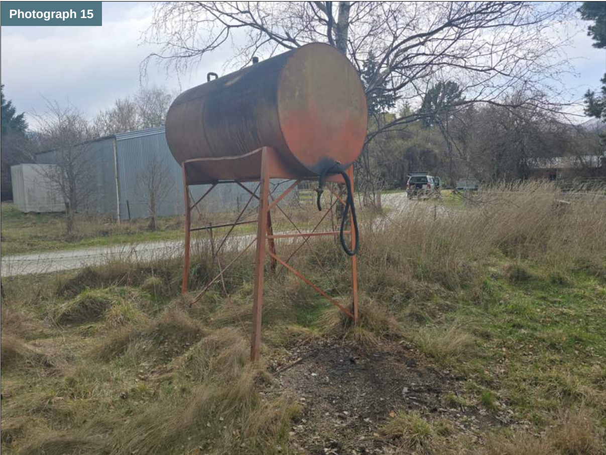
Aboveground storage tank with ground surface staining visible (Area 1)
