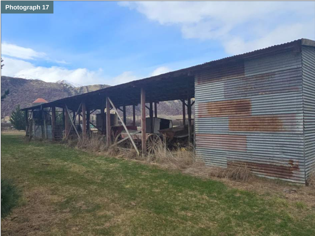
Farm implement shed east of the livestock holding sheds, of steel and timber construction, in poor condition. (Area 1)
