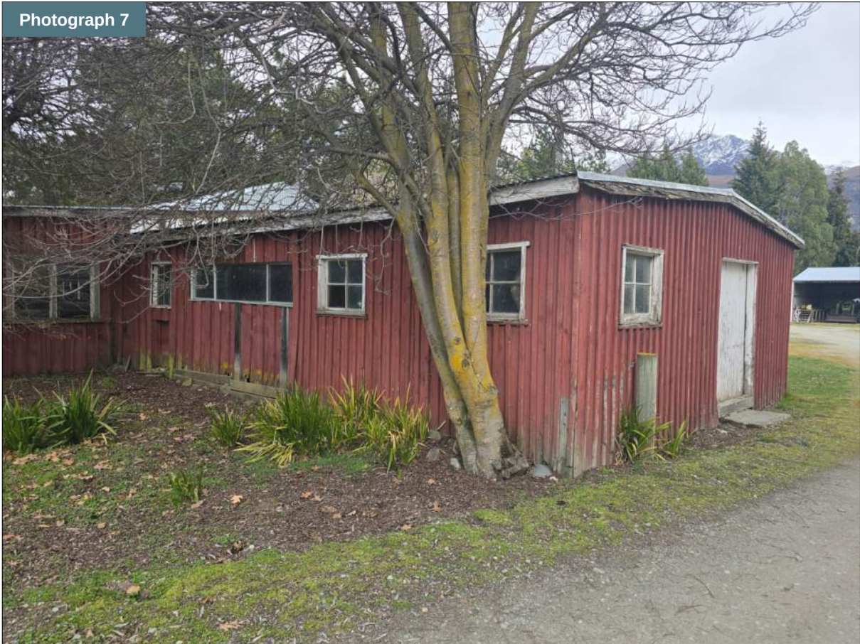
Painted exterior, deteriorated and flaking (Area 1)
