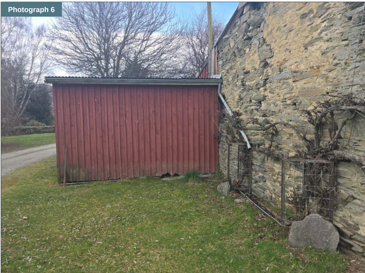
Painted exterior, deteriorated and flaking (Area 1)
