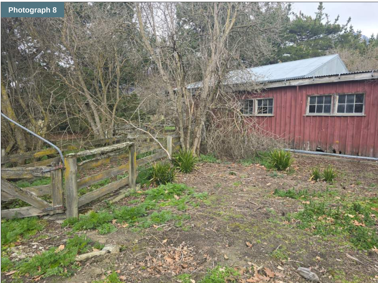
Livestock holding shed and pens, painted exterior, deteriorated and flaking (Area 1)
