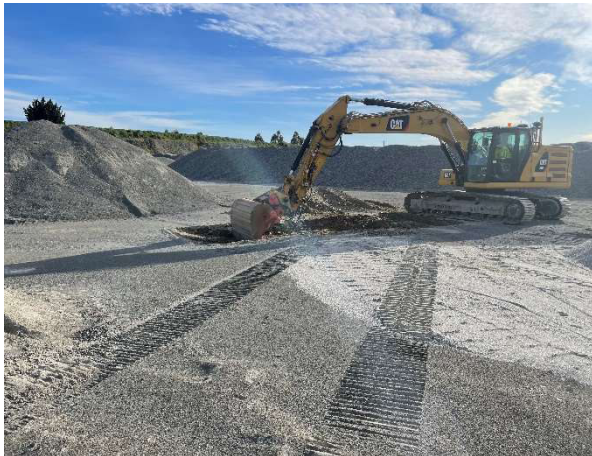
Photograph 3: Over-excavation of the base.
