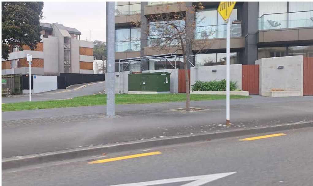
Figure 42 Berm side electrical transformer at 251 Victoria Street (western side of Karo Drive) 10/05/2026
