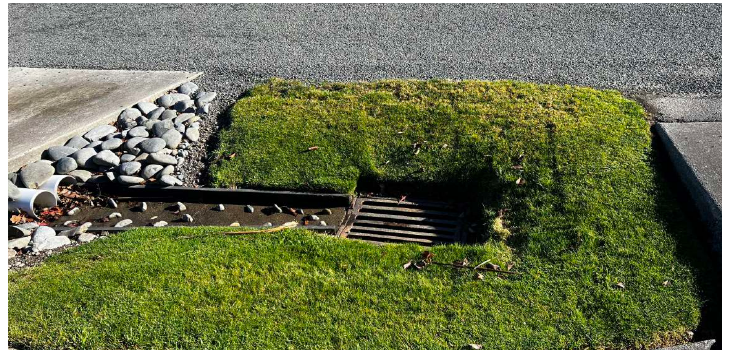
Swale drains: Swales are located within the road reserves along Mapleham Drive, T e Haunui Lane, Mara Kai Place and Atkinsons Lane.
