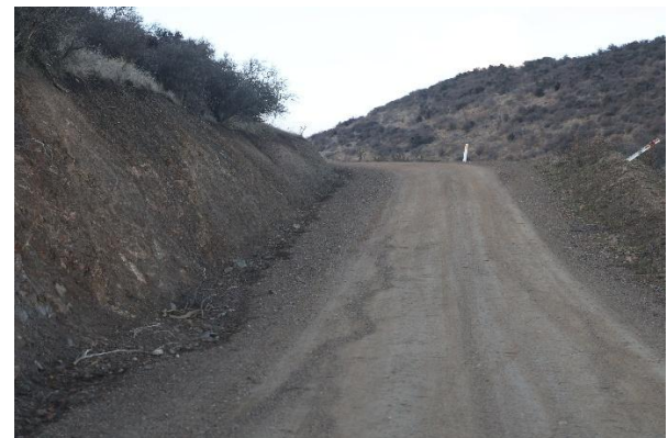
Figure 6: Surface rilling and road edge scour
