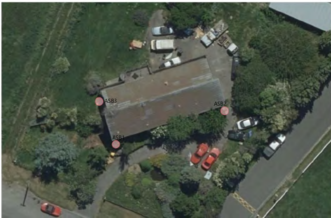
Figure H6: Asbestos containing roof material at 500 Avonhead Road
