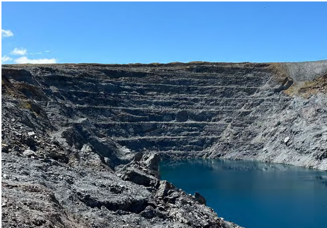
Inset 12: Condition of the Stage 4 East Wall in February 2025.
