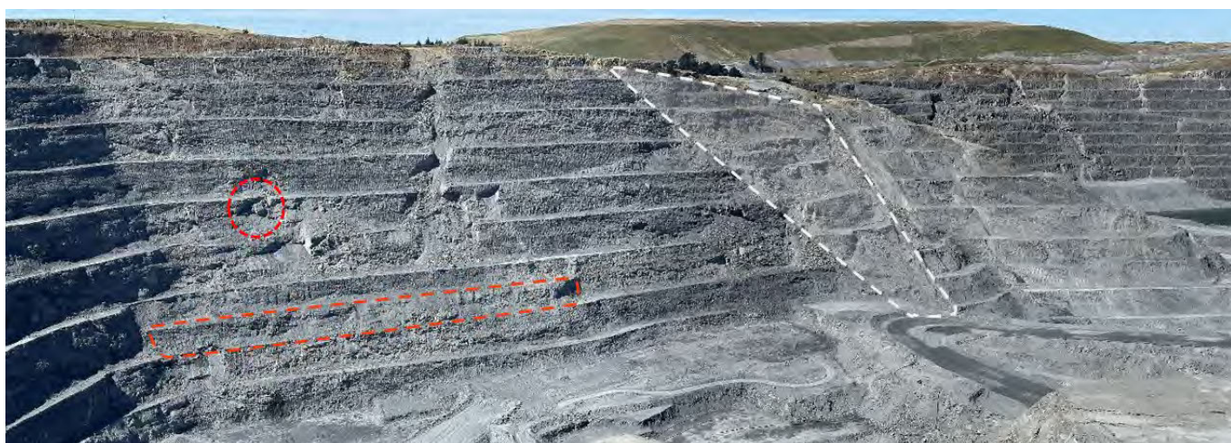
Inset 22: View of IM8 east wall. 430 mRL step off highlighted in orange. The extent of the southern instability highlighted in white.
