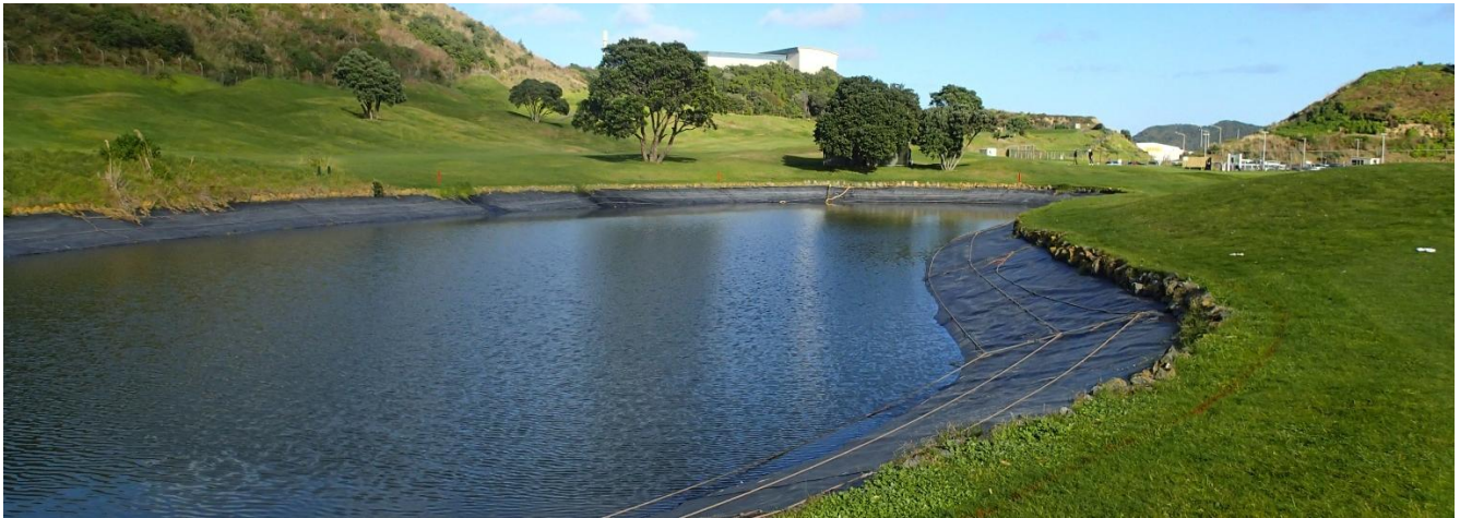
Photo 13. Water storage pond used for irrigation on Miramar Golf Course.
