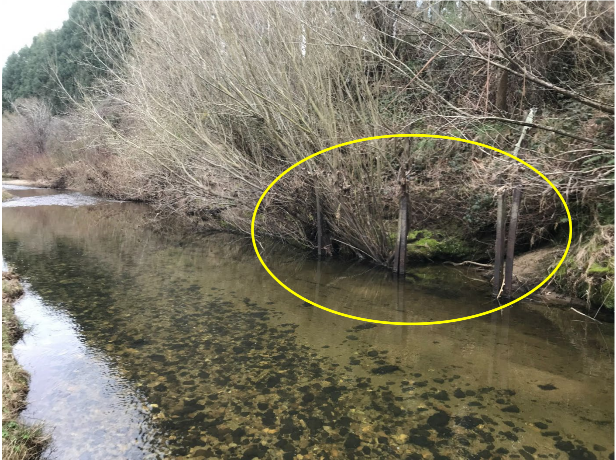
Figure 14. Railway iron (highlighted by a yellow circle) placed along the Silver Stream bank (photograph provided by e3 Scientific)
