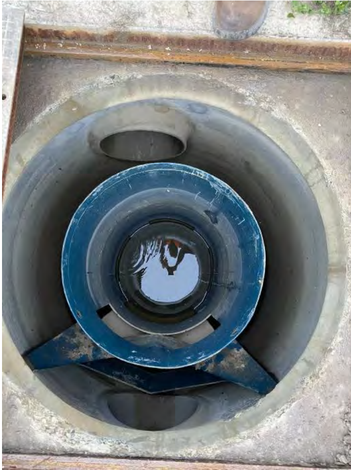
Figure 3-7: Typical proprietary GPT 3
