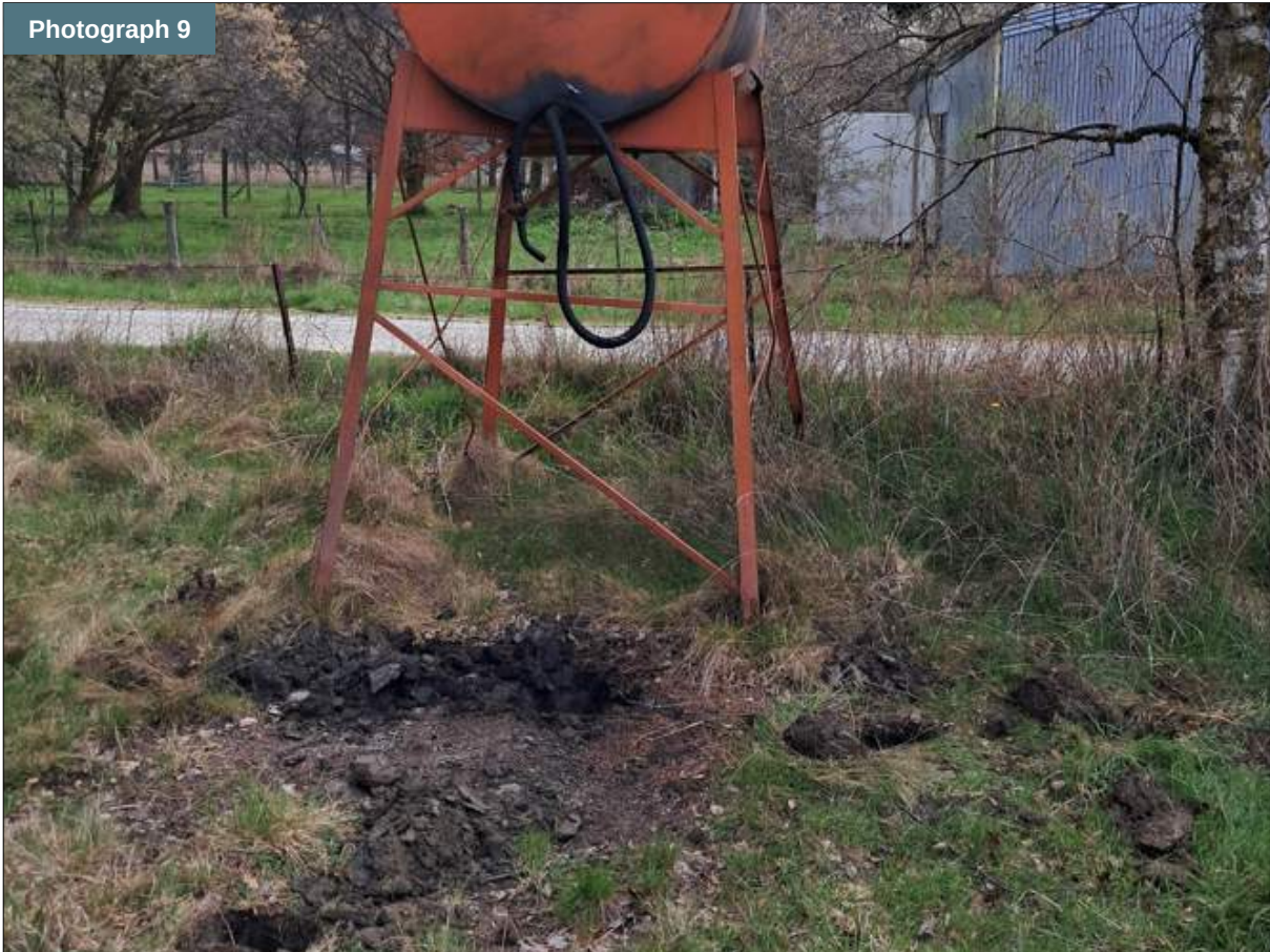
AST, with visible surficial soil staining below
