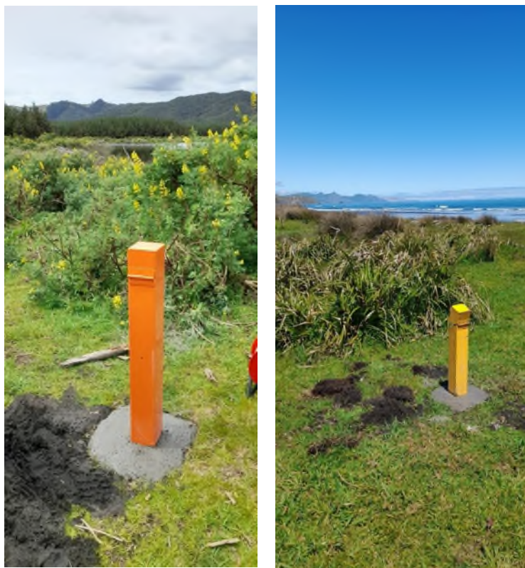
Figure 6. Piezometer installed in Wetland 72 (left) and Wetland 80 (right).
