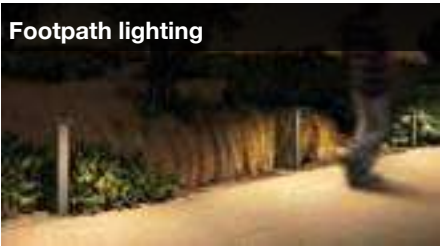
Low-glare entry and path lighting (bollards / low poles / wall-mounted at buildings), focused on routes and thresholds.
