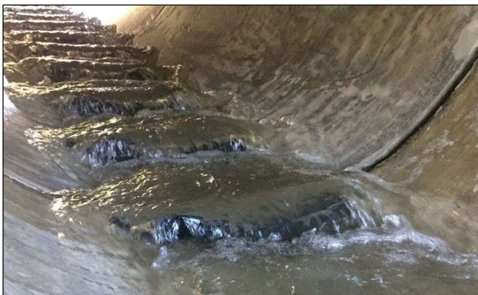
Plate 16: Example of a culvert with flexible baffles installed. The baffles alter the flow while providing rest areas for species travelling upstream.
