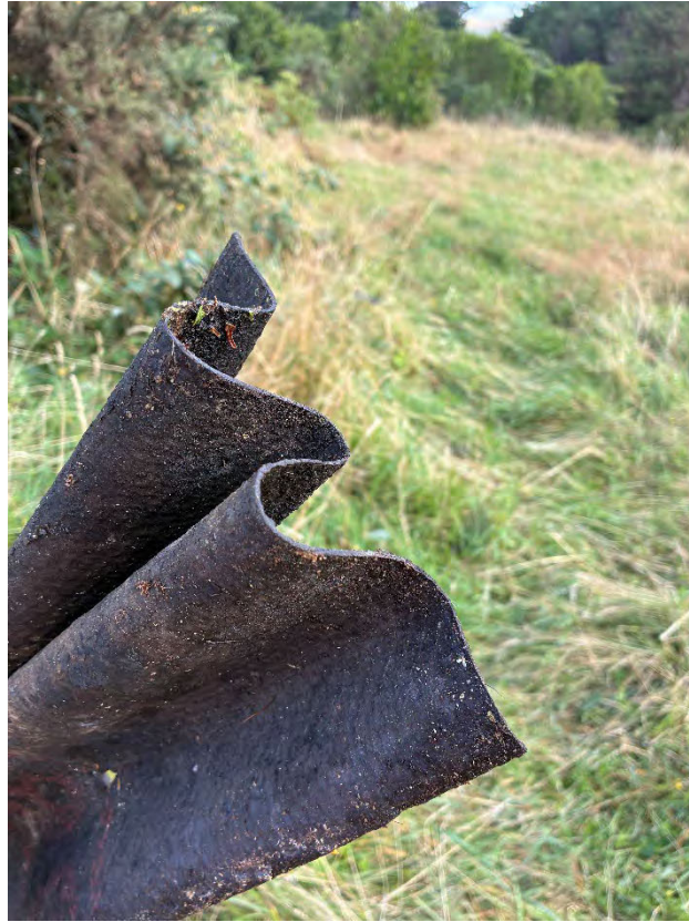
Photograph 7: Photo of potential asbestos at SS01.
